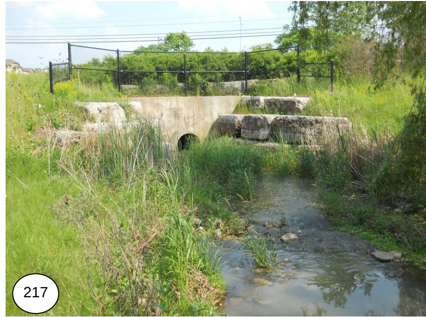
Online Pond control structure
