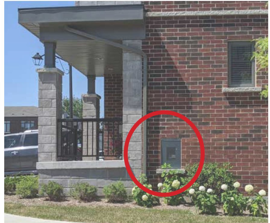
Fig. 6.4.7a - Utilities should be discreetly located, integrated into the architecture or screened from public view
