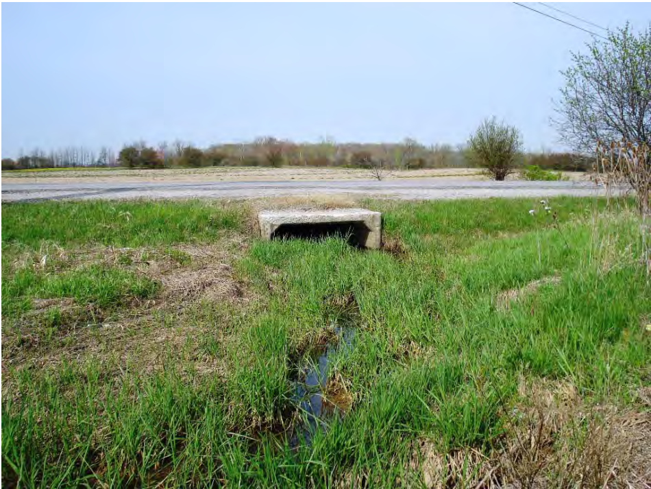
Photograph 4: Culvert located on the western portion of the Site, off Sixth Line.
