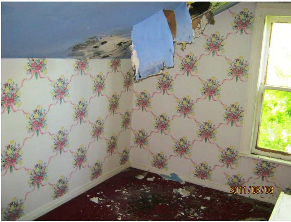
Photograph 15: General view of mould and ceiling water damage in the second floor of the house.
