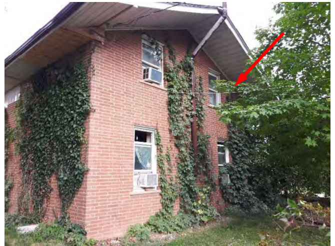
Photo 4: View of a portion of the southwest elevation (see arrow) of the Subject Building, looking southeast.
