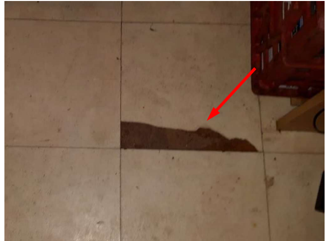
Photo 12: View of a damaged vinyl floor tile (see arrow) in the kitchen of the Subject Building.
