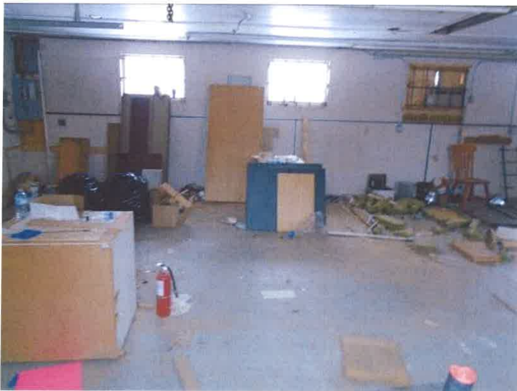
View of the interior of garage at 2460 Old Bronte Road (facing south)
