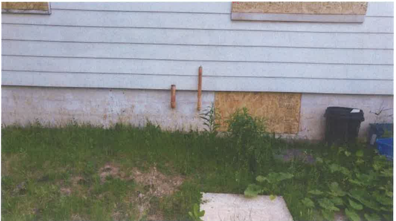
Vent and filler pipe for the ASTs at 2444 Old Bronte Road (facing northeast)
