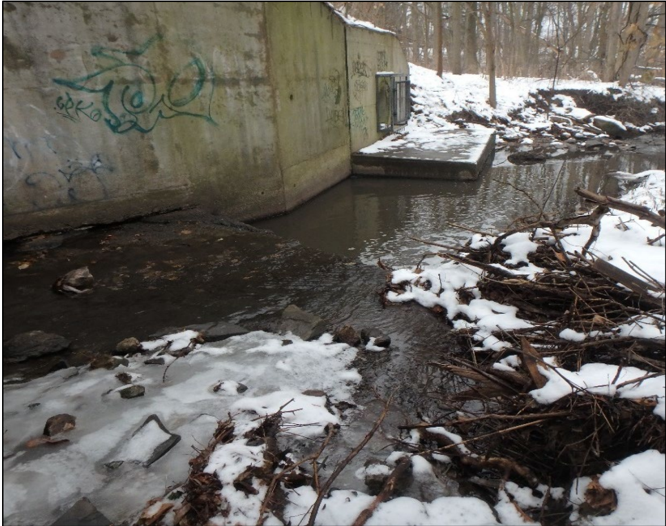
Figure 3-17: Fish Barrier at Rebecca Street Crossing
