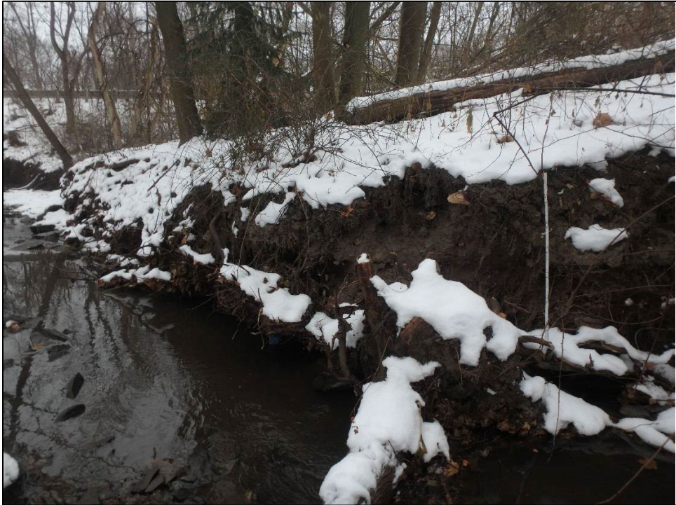
Figure 3-19: Erosion along West Bank of McCraney Creek
