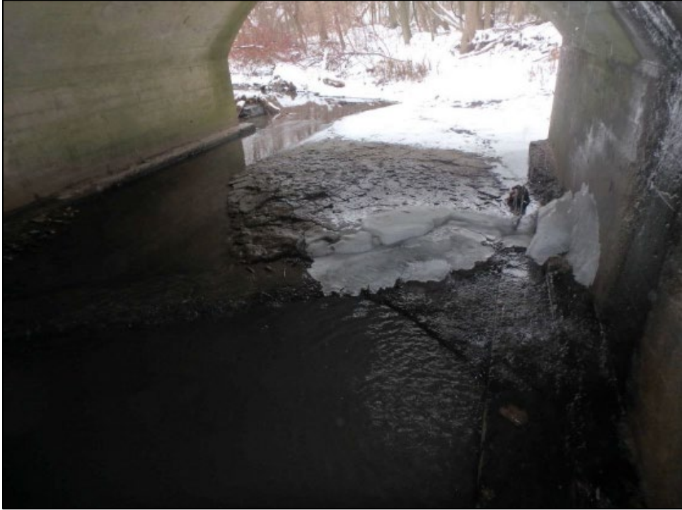
Figure 3-20: Fish Barrier at Lakeshore Road Crossing
