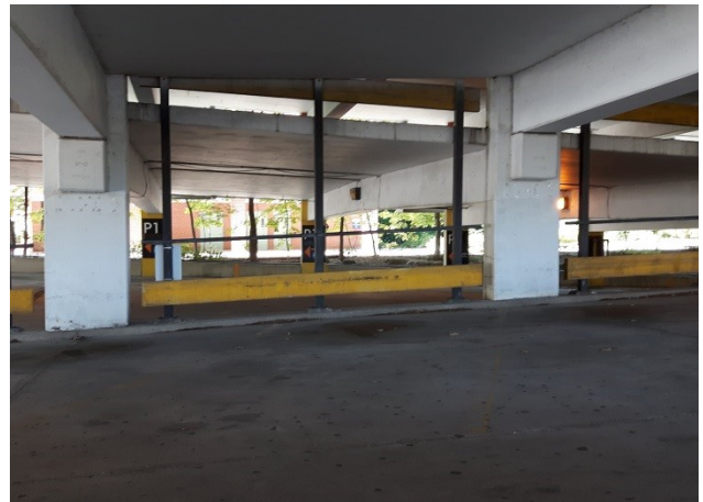
Photo 16: View of the interior of the parking garage located in the central portion of the Site property.
