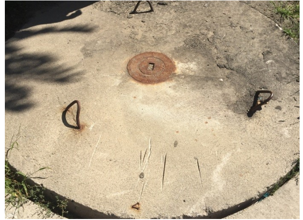
Photo 14: View of the chemical storage tank located at the western portion of the former hospital building exterior.
