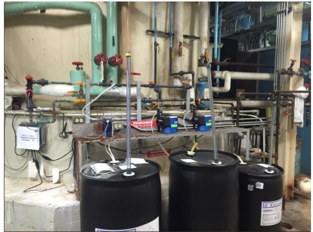
Photo 4: View of the water treatment system located in the basement of the former hospital.
