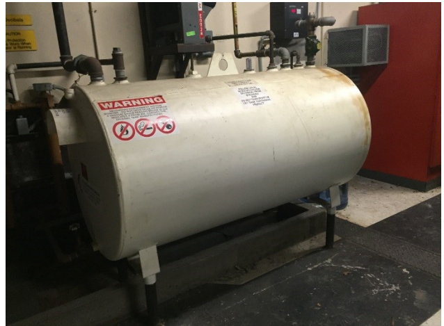
Photo 6: View of the diesel AST located in the diesel generator room of the former hospital.
