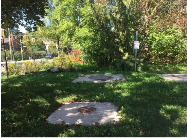
Photo 13: View of the USTs located at the northwest corner of the Site property).
