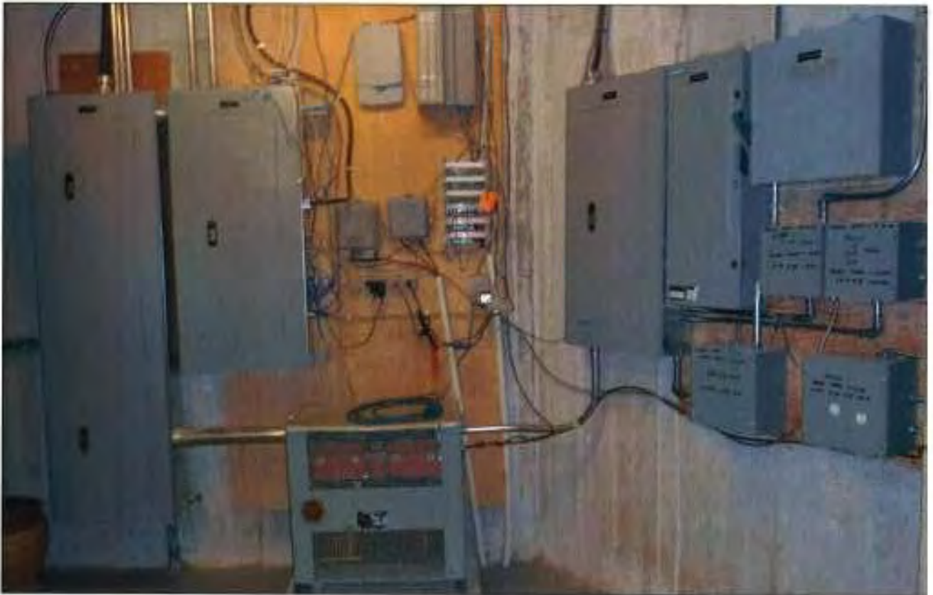
Photograph 11 View of the Electrical Equipment in the Basement
