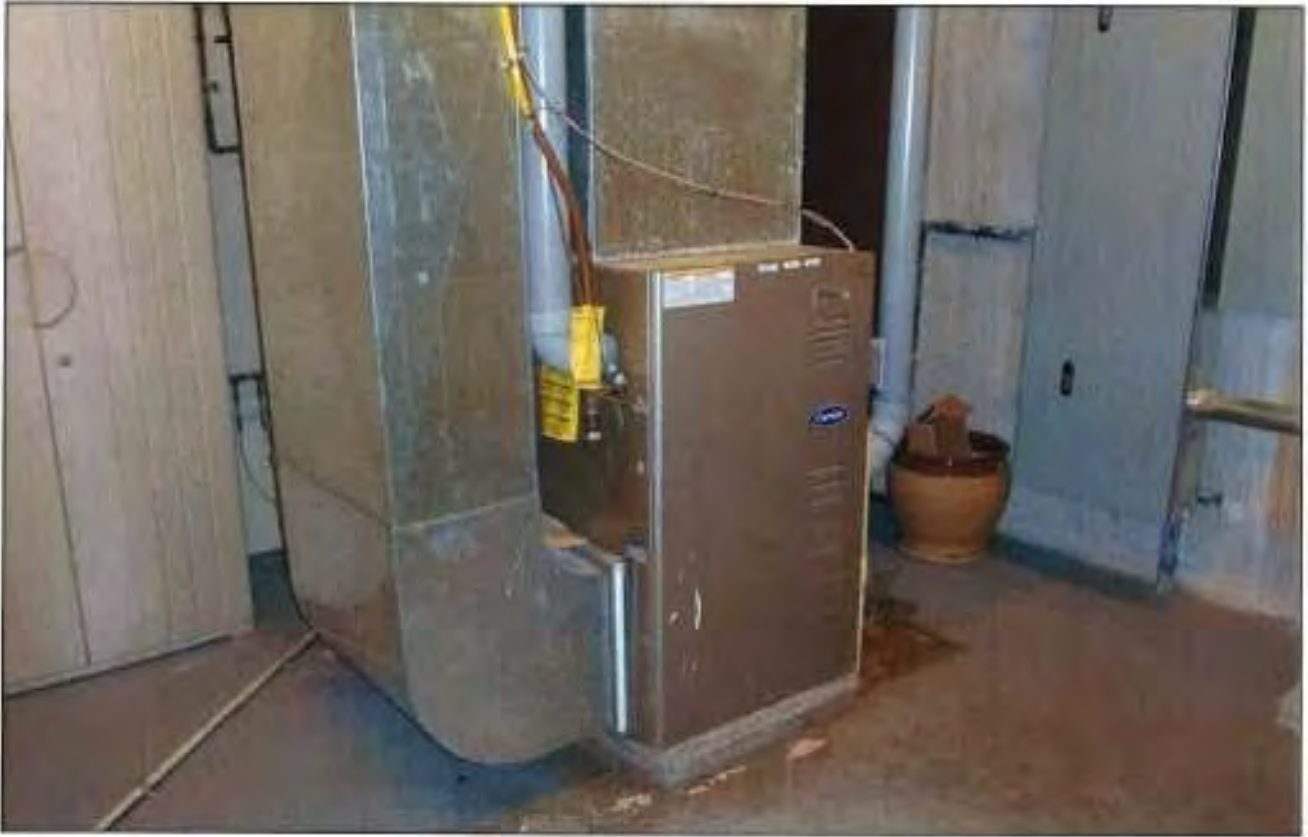
Photograph 10 View of the Propane-Fired Carrier Furnace in the Basement
