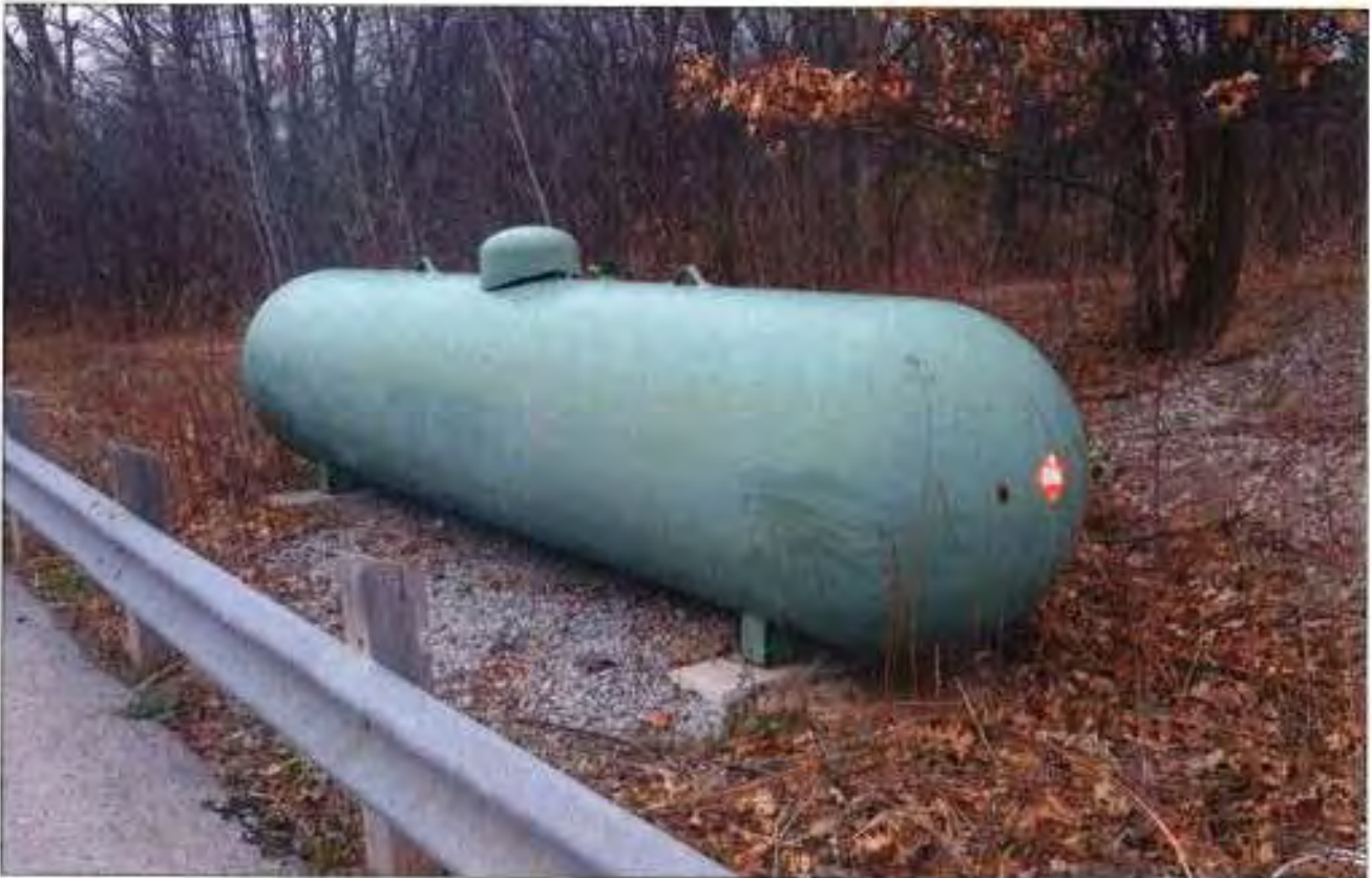
Photograph 15 View of Propane AST on the Western Portion of the Site
