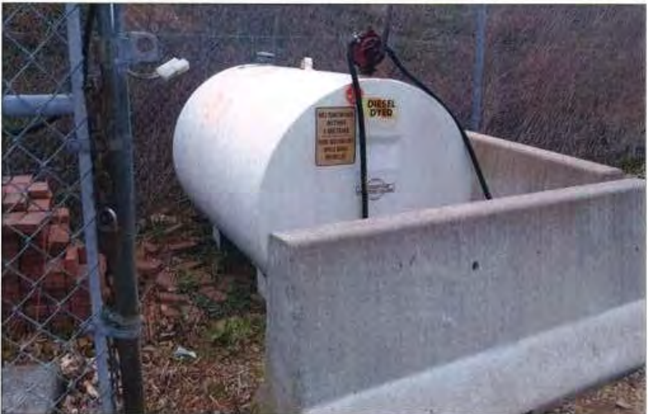
Photograph 21 View of Diesel AST in Maintenance Yard
