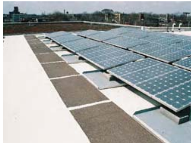
Photo 3.32: This lightly coloured cool roof has some of the benefits of a green roof and integrates photovoltaic cells to supplement the building energy needs.
