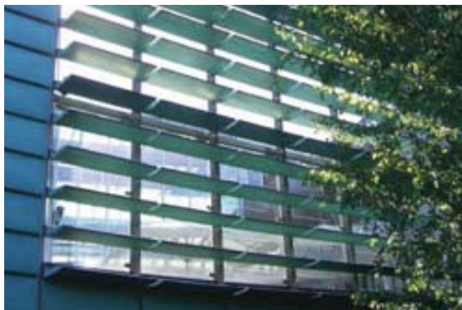
Photo 3.28: Louvers control direct sunlight and maximize desirable indirect daylighting.
