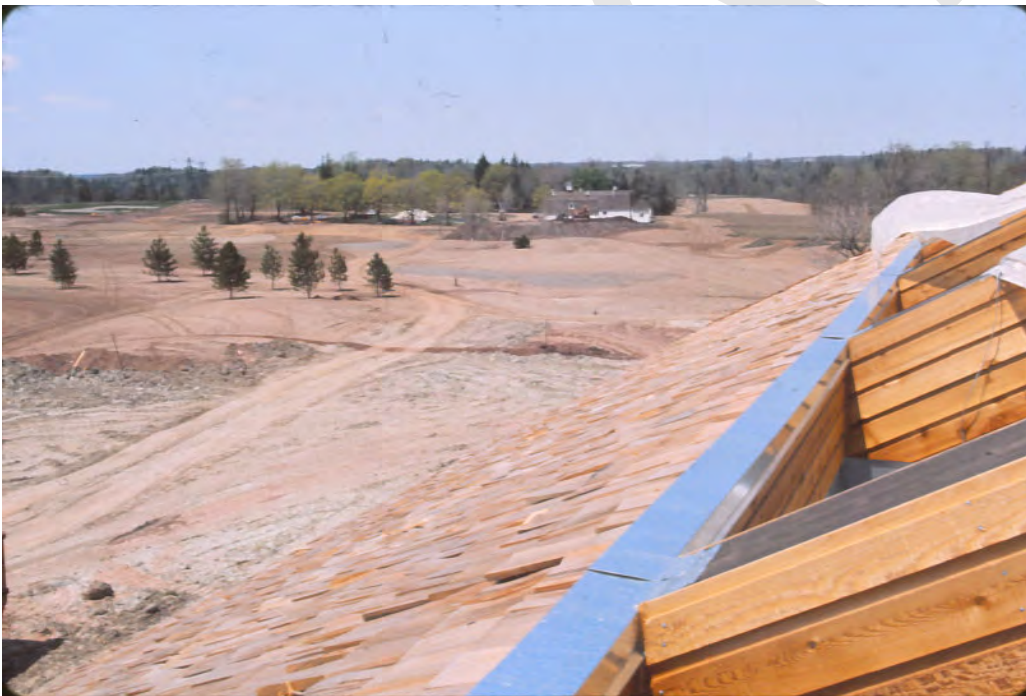
Figure 19: View of golf course construction from clubhouse, [c.1976] (Golf Canada Museum Archives).
