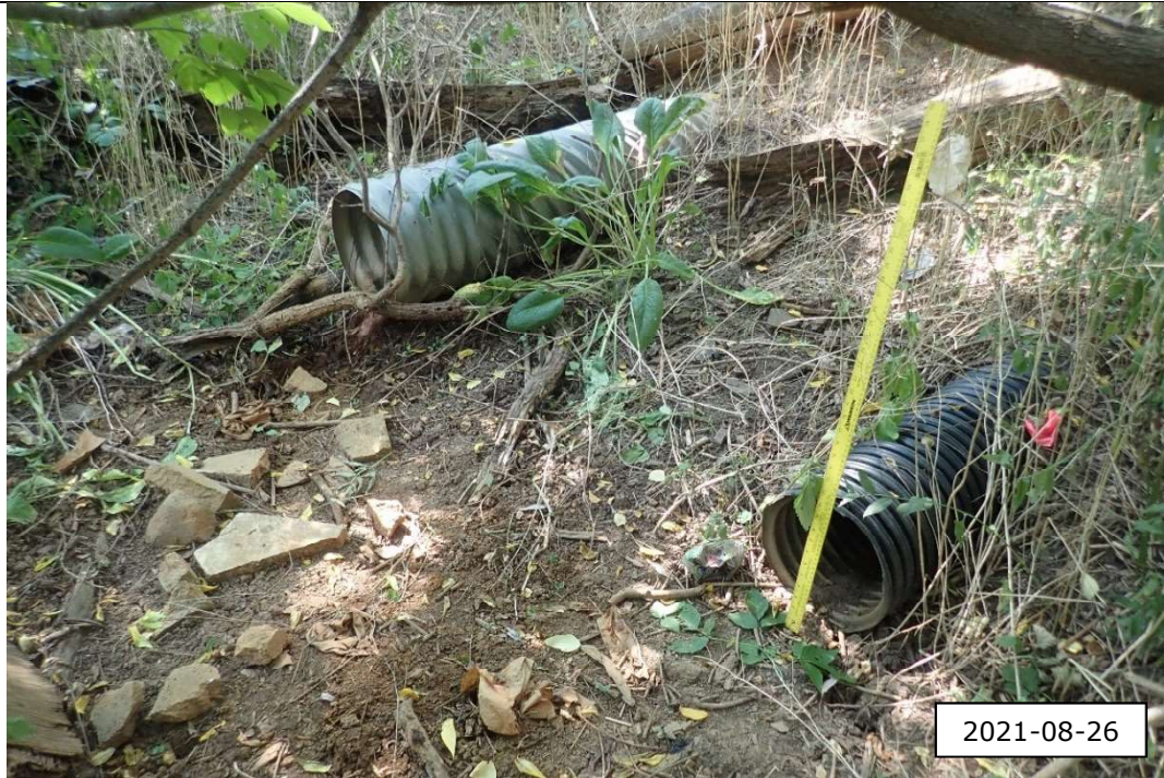
Upstream view towards the upstream extent of the ravine feature. The two culverts, left to right, were approximately 0.40 m and 0.30 m in diameter.
