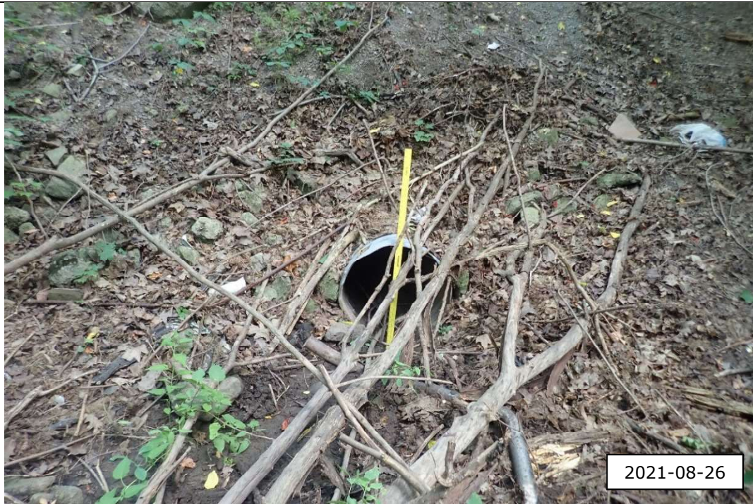
Photo taken at the downstream extent of reach, facing downstream. The culvert connected to Reach GC2 and was approximately 0.5 m in diameter.
