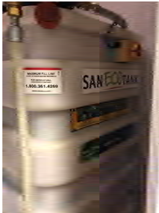
Photo 6: Grease container located on the north portion of the Site building.
