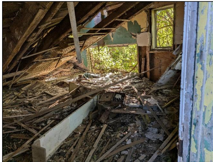
Photograph 5: Collapsed Floor on South Side of the House
