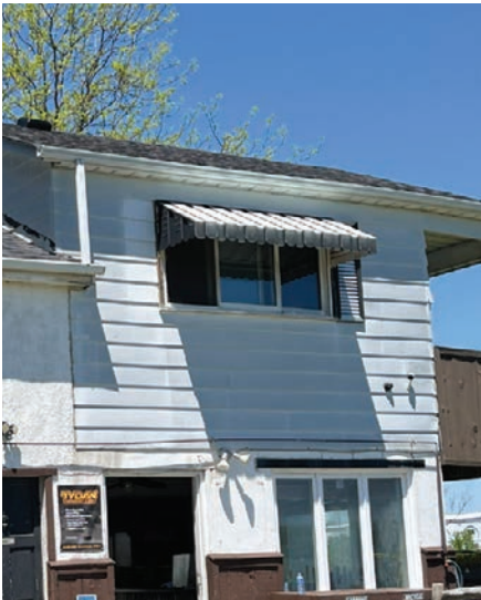
Metal siding in fair condition, with areas of poor condition (ERA, 2025).
