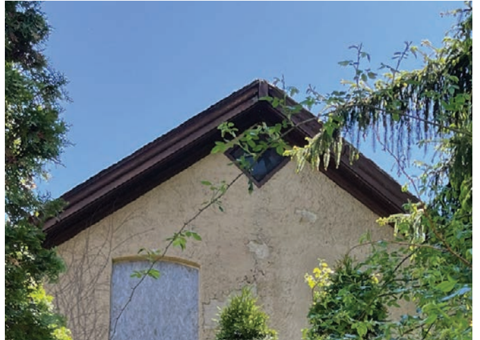
Wood fascia in poor condition (ERA, 2025).
