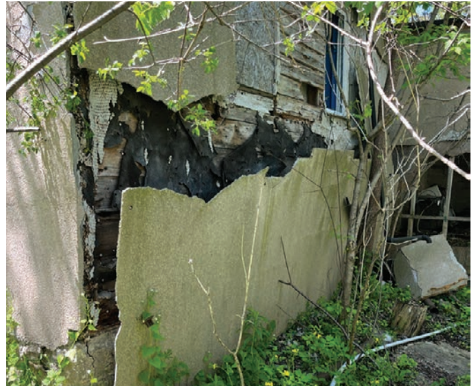
Areas of stucco in defective condition (ERA, 2025).
