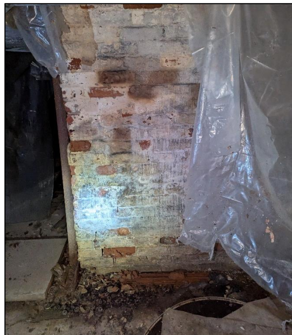
Photograph 12: Brick Spalling and Deterioration at Base of Interior Foundation Wall
