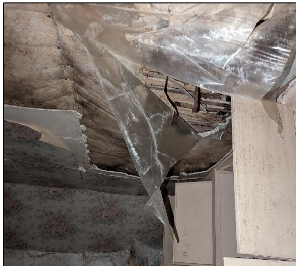
Photograph 2: Example of Water Damage of 2 nd Floor Ceiling
