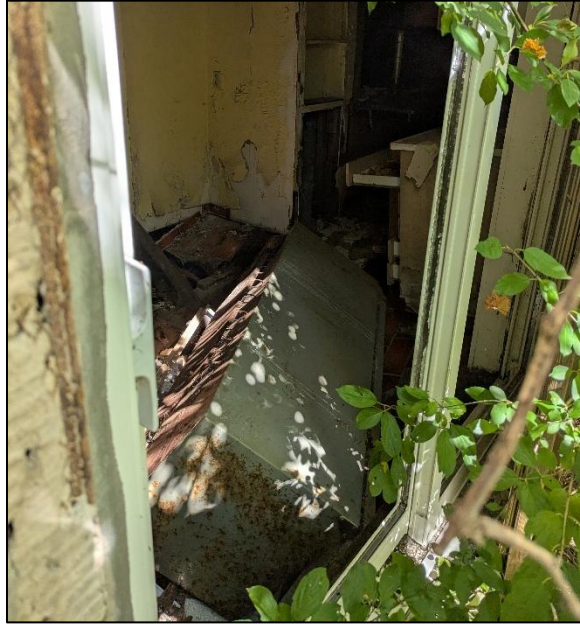
Photograph 18: Broken Sliding Glass Door on South Side of South Addition
