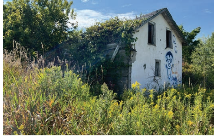
Stucco missing from entirety of rear (east) elevation (ERA, 2025).
