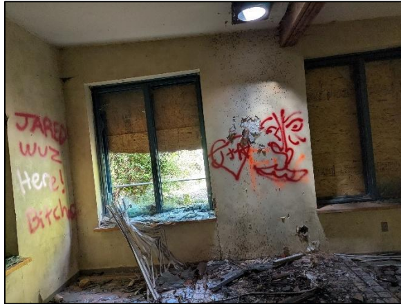
Photograph 19: Damaged Board Over Opening on Main Floor of North Addition
