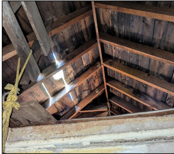
Photograph 1: Hole in Roof of Original Building
