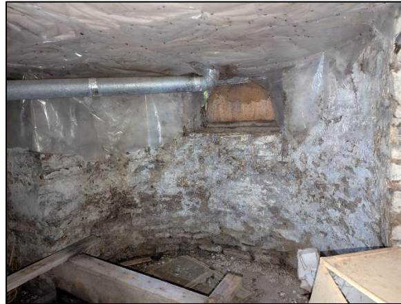
Photograph 11: Mortar Deterioration at Bottom of Stone Foundation Wall
