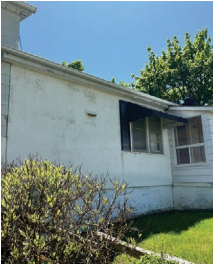
Stucco in poor condition (ERA, 2025).
