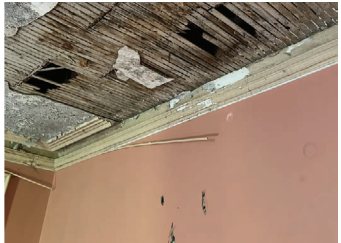
Plaster cornice in poor to defective condition (ERA, 2025).
