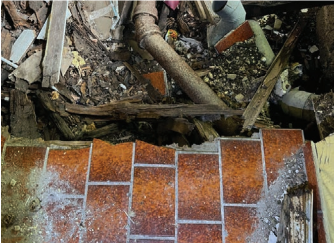
Tile floors at the later addition in defective condition (ERA, 2025).
