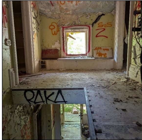
Photograph 5: Boarded Window with Damage on Second Floor
