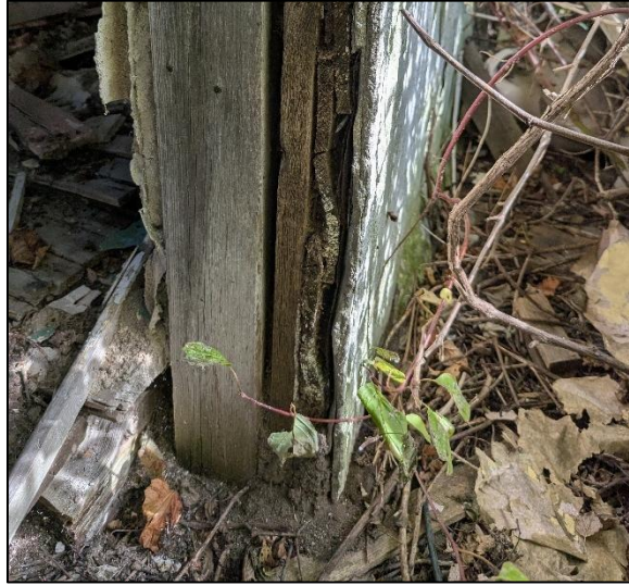
Photograph 1: Exterior Stud Below Grade & Wood Rot at Base
