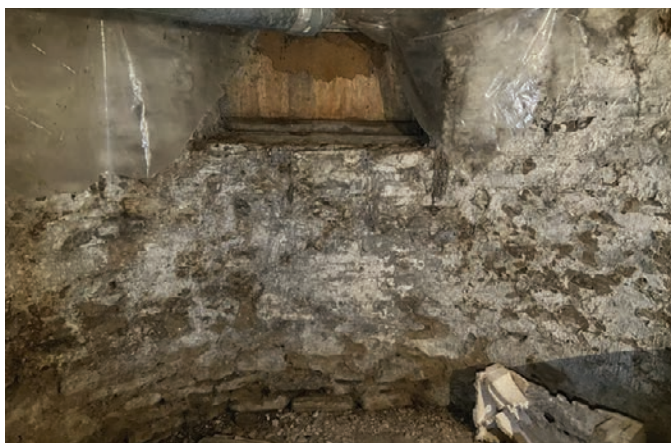
Fieldstone foundations, viewed from the basement, in poor condition (ERA, 2025).
