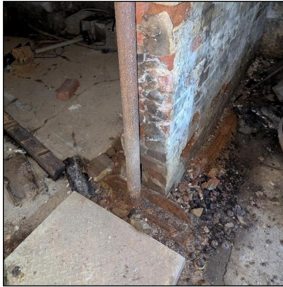
Photograph 7: Severe Corrosion at Base of Steel Telepost
