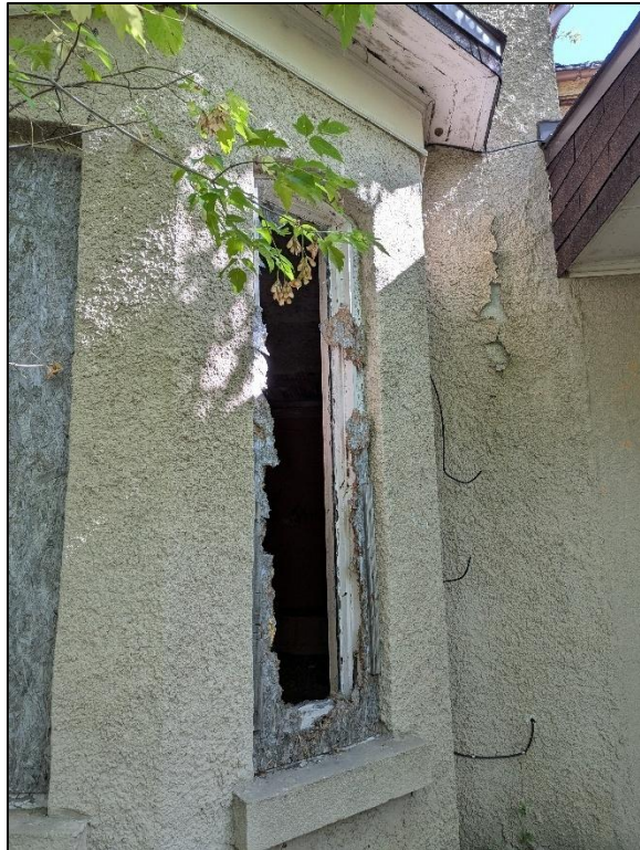
Photograph 4: Boarded Window with Damage Allowing Access to Interior
