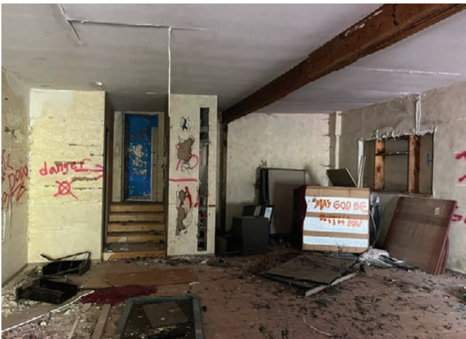
Ceiling at the north part of the later addition in poor condition (ERA, 2025).
