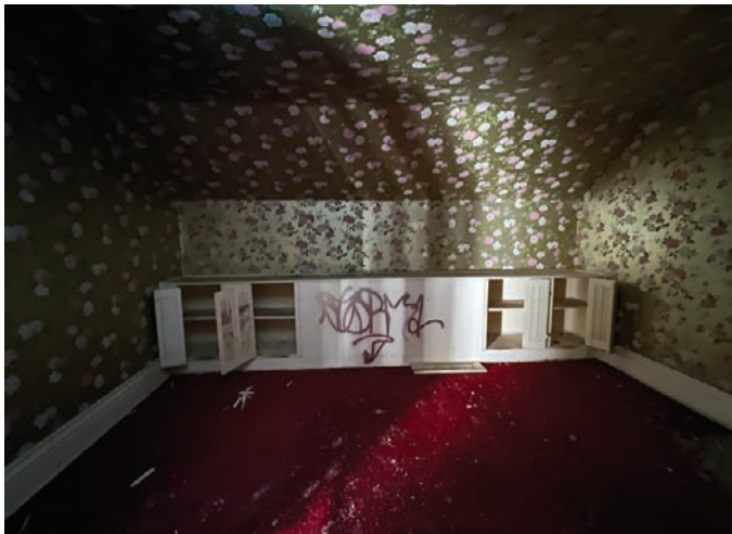
Carpet floors at the second floor in poor to defective condition, with extensive water damage (ERA, 2025).
