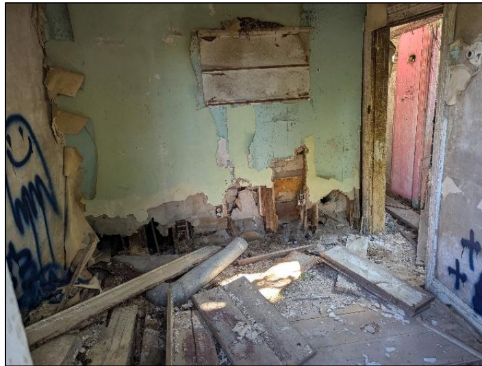
Photograph 7: Damage at Base of Interior Walls
