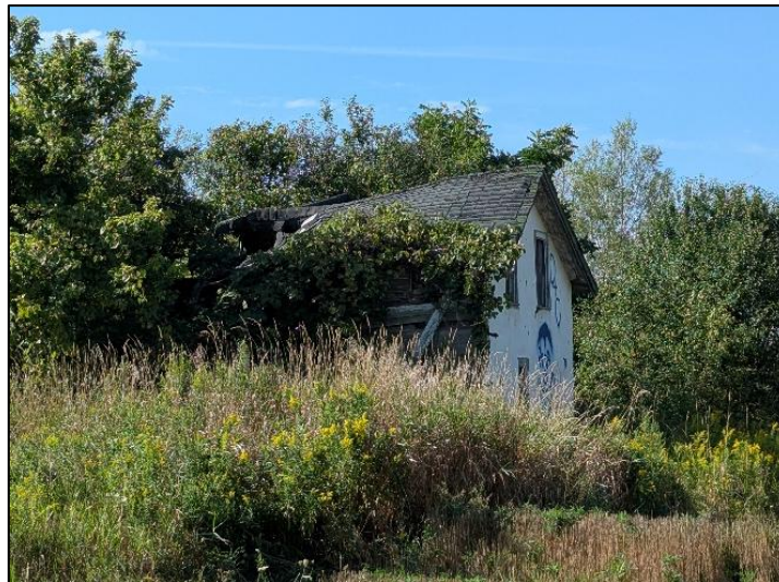
Photograph 4: Collapsed Roof on South-East Corner of House
