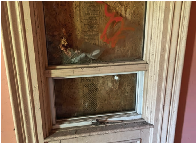
Window in defective condition, with extensive missing glazing (ERA, 2025).
