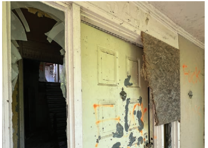
Main entry door in poor condition with sidelights in defective condition with broken glazing (ERA, 2025).
