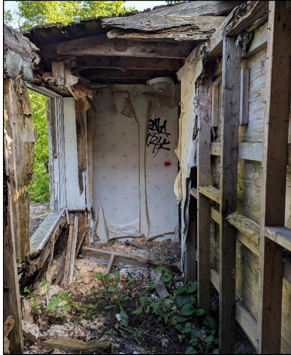
Photograph 13: Collapsed Roof of South Side Addition
