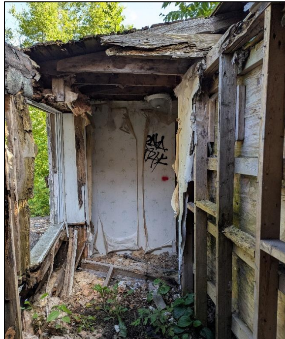
Photograph 21: Rot of Second Floor Wall Studs in South Addition
