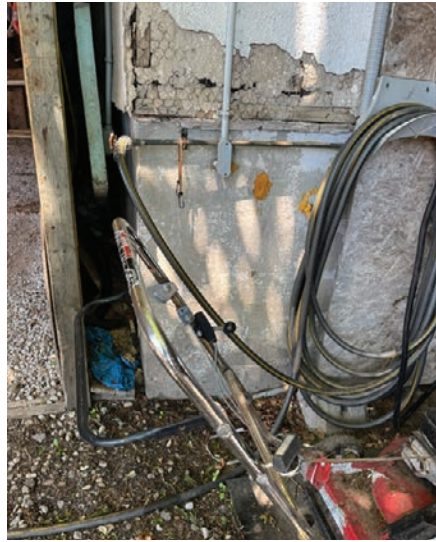
Stucco in poor condition, showing delamination (ERA, 2025).
