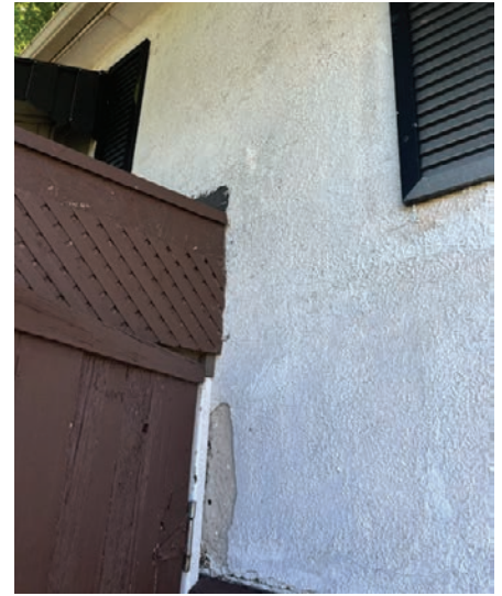
Stucco in poor condition, showing cracking and delamination (ERA, 2025).
