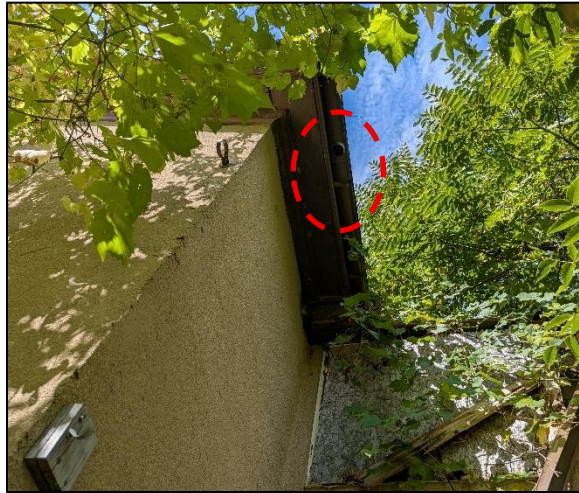
Photograph 3: Example of Downspout Disconnected from Eavestrough
