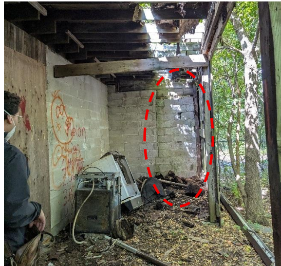
Photograph 24: Concrete Block Wall in Poor Condition at Northeast Corner
