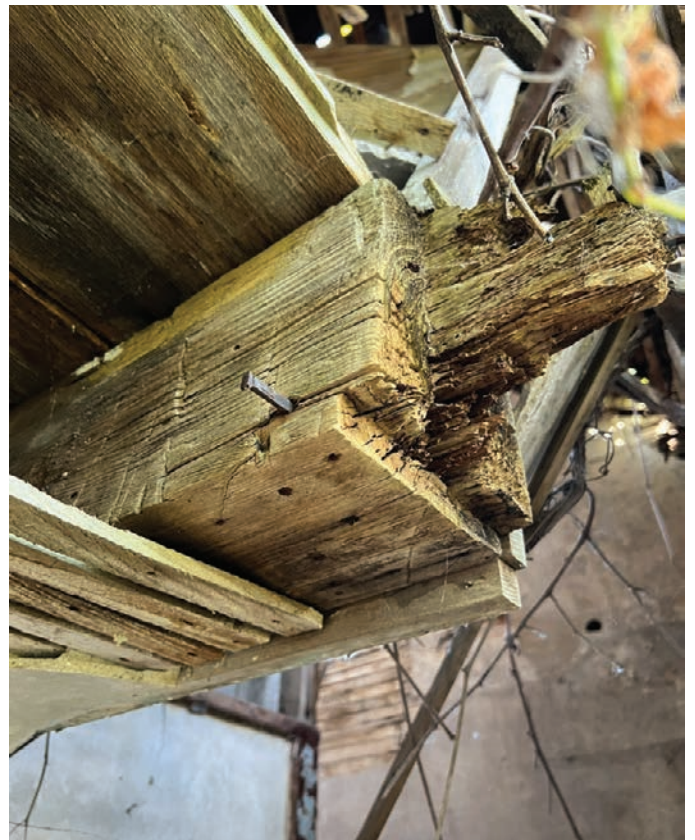
Beam tenon on the east elevation where the mortise-and-tenon connection has failed (ERA, 2025).
