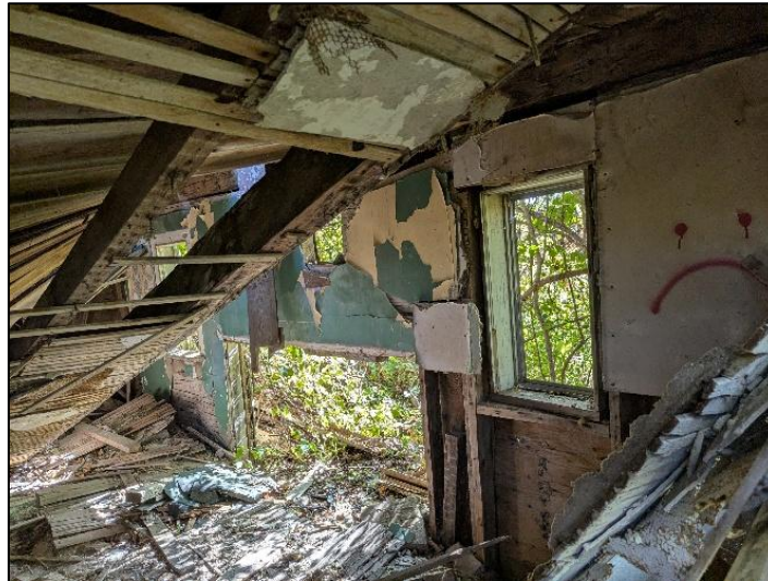
Photograph 2: Missing Chimney Walls and Broken Windows on South Elevation
