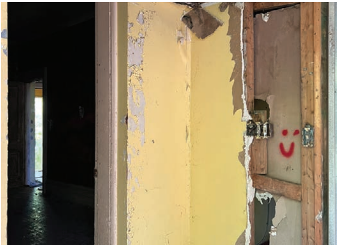
Drywall at the later addition in poor to defective condition (ERA, 2025).
