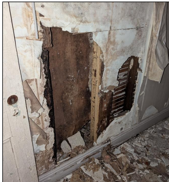
Photograph 6: Rot of Interior Wood Stud Wall Below Hole in Roof
