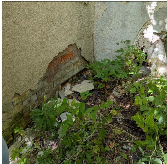
Photograph 8: Brick Spalling at South-East Corner of Original House
