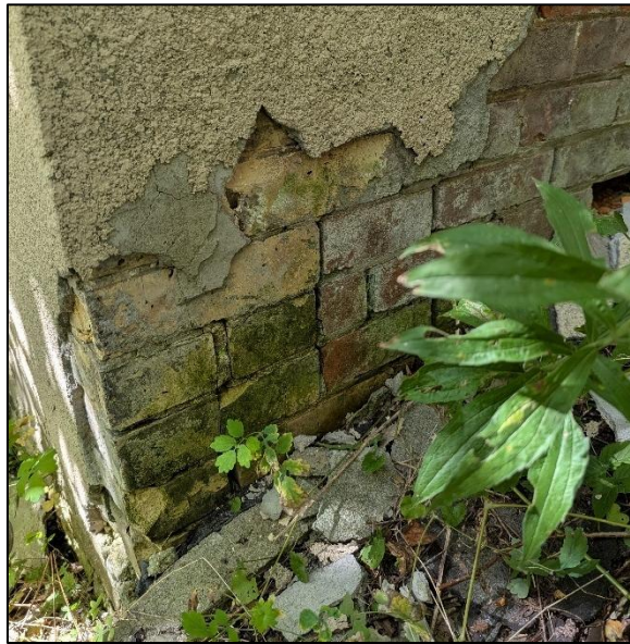
Photograph 10: Mortar Deterioration in Masonry Wall
