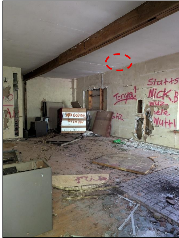
Photograph 15: Water Staining of North Addition Ceiling
