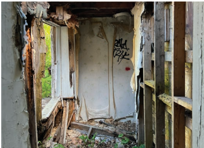
The roof of the south portion of the later addition is partially collapsed (ERA, 2025).
