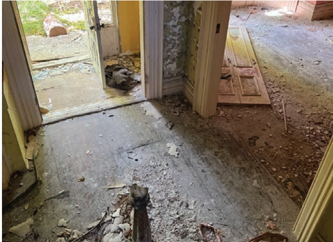
Floors at the original portion of building in fair to poor condition (ERA, 2025).
