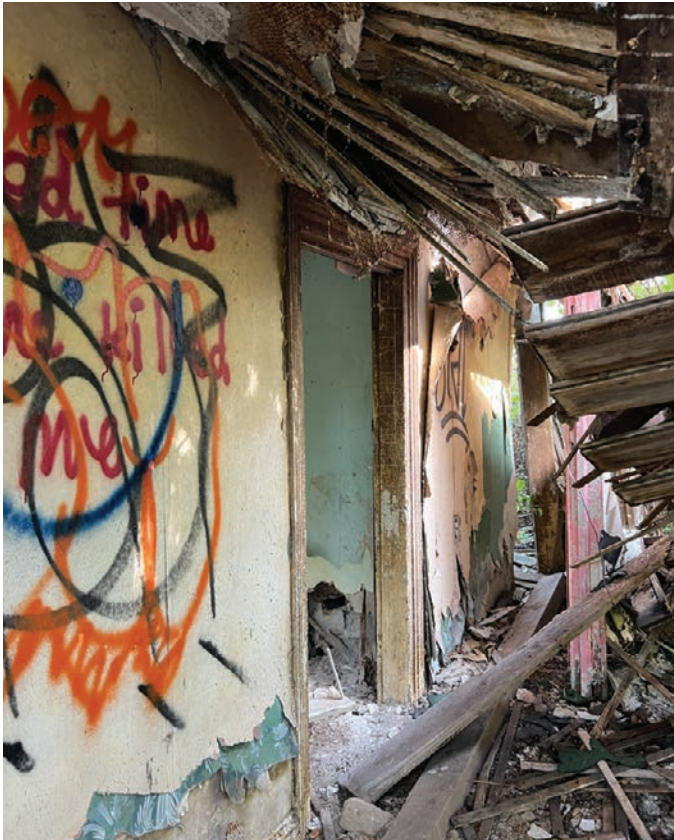
Collapsed roof on the first storey, looking northeast from the main entrance (ERA, 2025).
