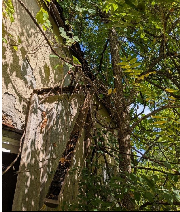
Photograph 17: Detached Eavestrough and Overgrown Trees
