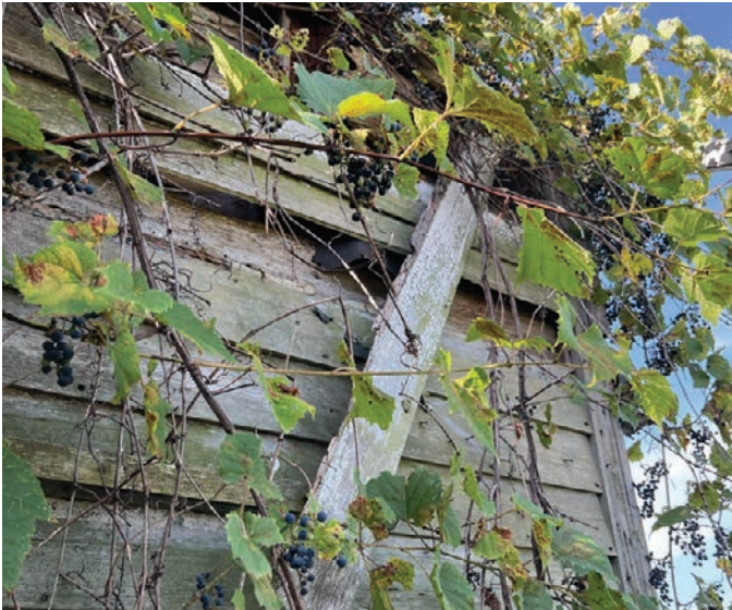
Close-up photo of rear (east) elevation wall, where the absence of stucco reveals the wooden siding and sheathing underneath which is in defective condition (ERA, 2025).
