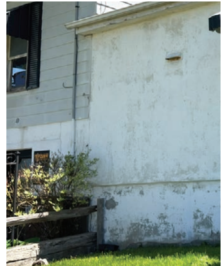
Concrete block wall mostly in fair condition despite defects (ERA, 2025).
