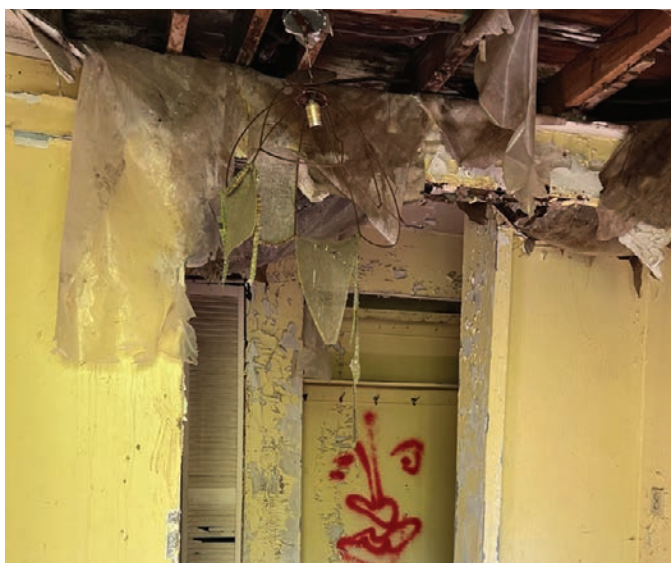
Interior spaces showing missing and damaged finished, revealing materials underneath (ERA, 2025).
