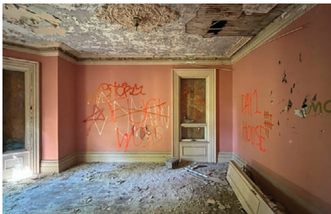
Interior spaces generally in defective condition (ERA, 2025).
