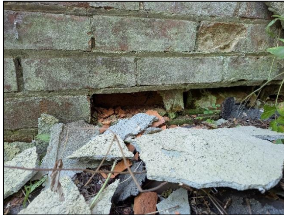
Photograph 9: Very Severe Masonry Deterioration at Grade
