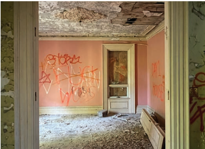
Wood trim at original portion of building in fair condition (ERA, 2025).
