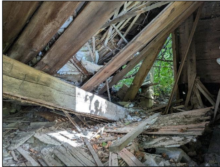
Photograph 3: Collapsed Exterior Wall on East Elevation
