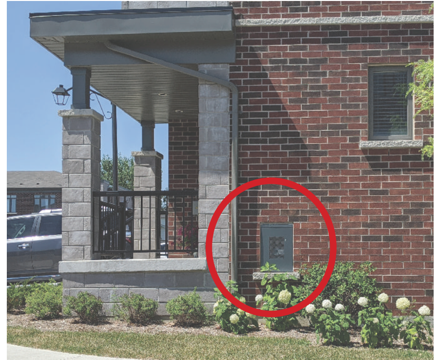
Fig. 7.6 - Utilities should be discreetly located, integrated into the architecture or screened from public view
