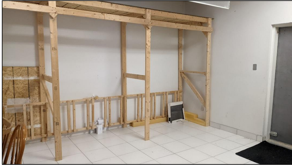
Photo 17: The northwest wall in the back room of the vacant unit (2365B Lakeshore Road West). looking north. .
