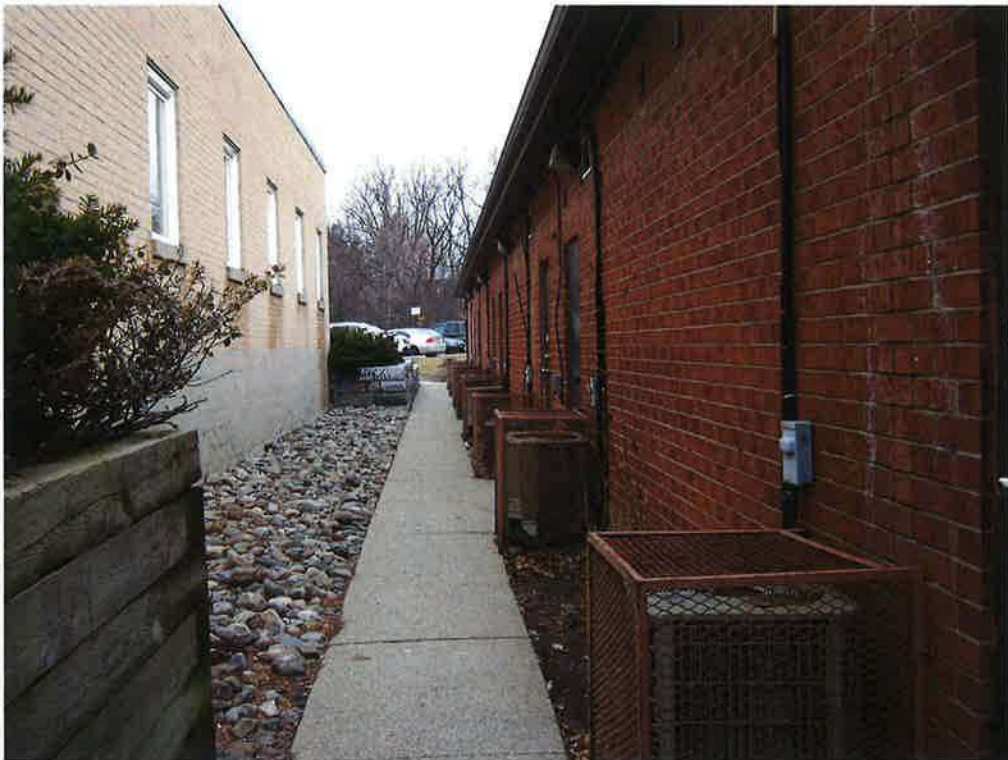
Air conditioning units (Looking north)
