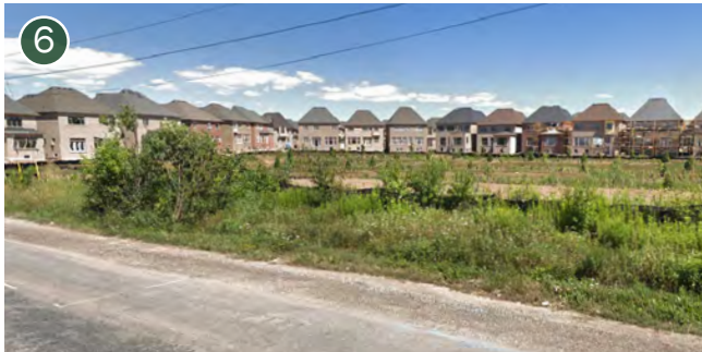
Existing single detached houses under construction backing onto NHS channel along east side of Sixth Line, south east of the Argo West Morrison subject lands.
