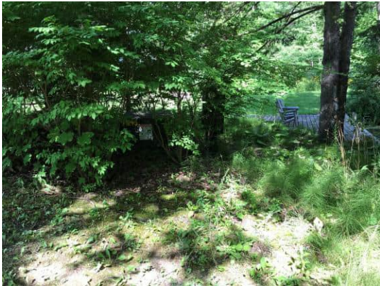
Picture 31: View of one (1) transformer located east adjacent to pond 2 (July 20, 2020).
