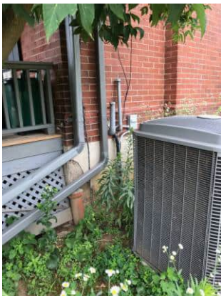
Picture 27: View of the vent pipes for the AST located at the basement of 1326 Bronte Road (July 20, 2020).
