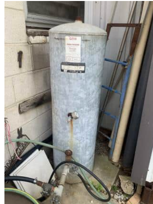
Picture 44: The pressurized water tank (used for irrigation of the garden) near the work shed at 1350 Bronte Road (July 21, 2021).
