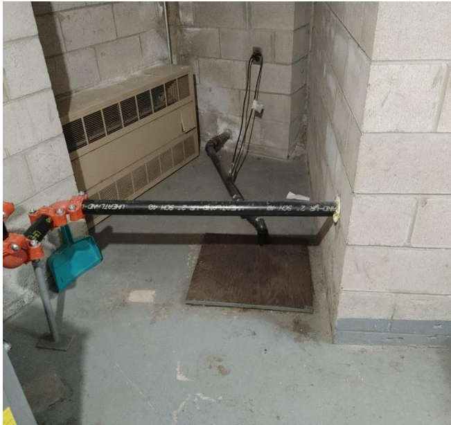
5- View of the sump pit and electric heater located in the lower-level elevator room
