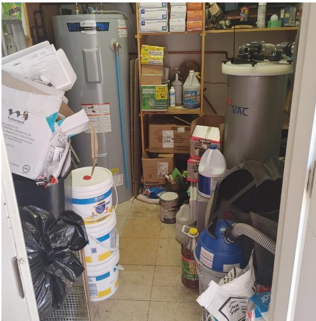
5- View of the maintenance room located in 587 Argus Road (Family Dentist Tree)
