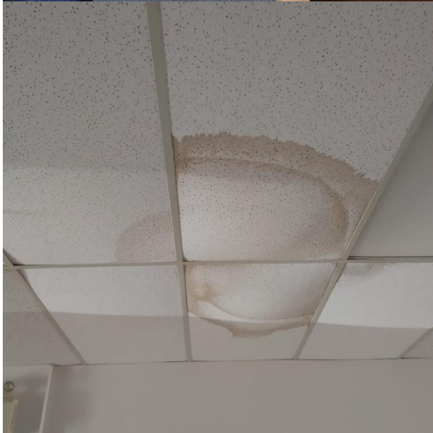
9- View of the moisture staining on the ceiling tile in 593 Argus Road (Vacant Unit)
