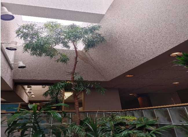
4- View of the moisture staining on the ceiling near the skylight in 587 Argus Road (Family Dentist Tree)
