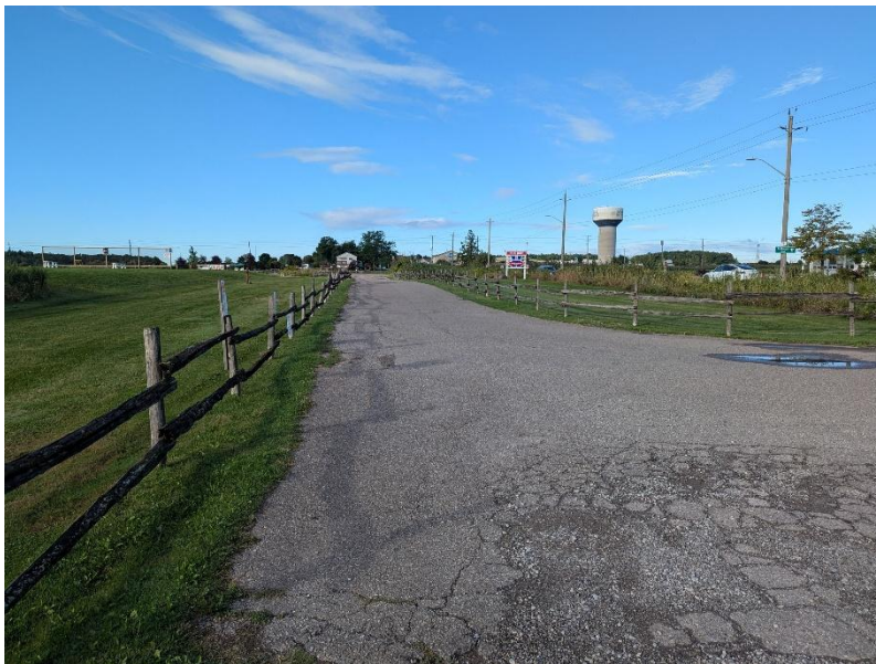
Image 12: View of the paved driveway and parking lot in the north of the study area.
