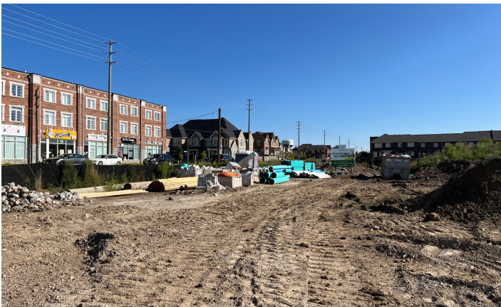
Photo 5: Storage of pipes, lumber, and bricks along northern corner of Site, facing north.
