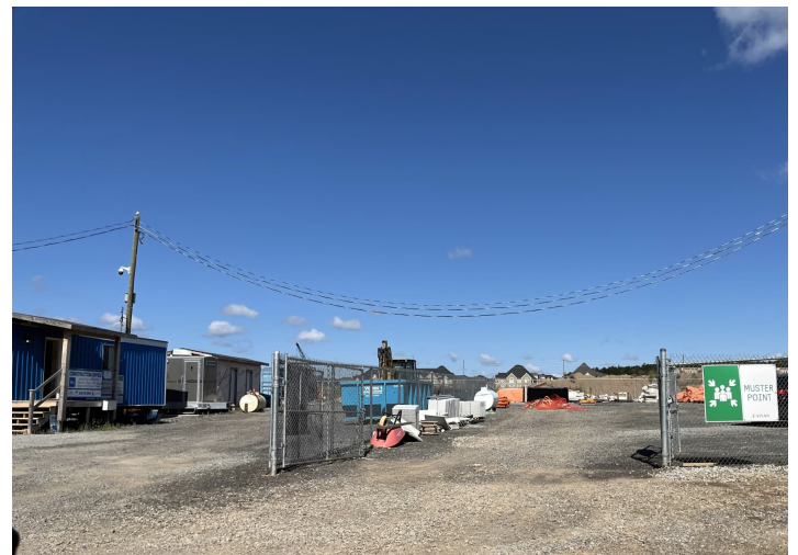
Photo 10: Two ASTs observed within fenced area of neighbouring construction, facing northwest.
