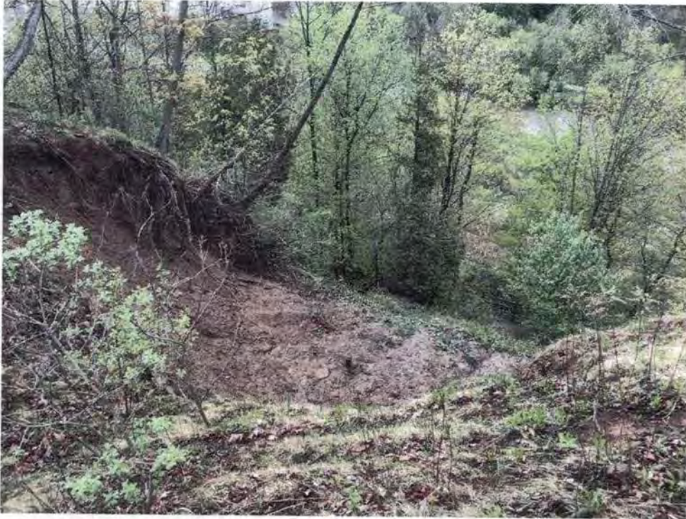
Sixteen Mile Creek Slope – Slope overburden erosion, looking East
