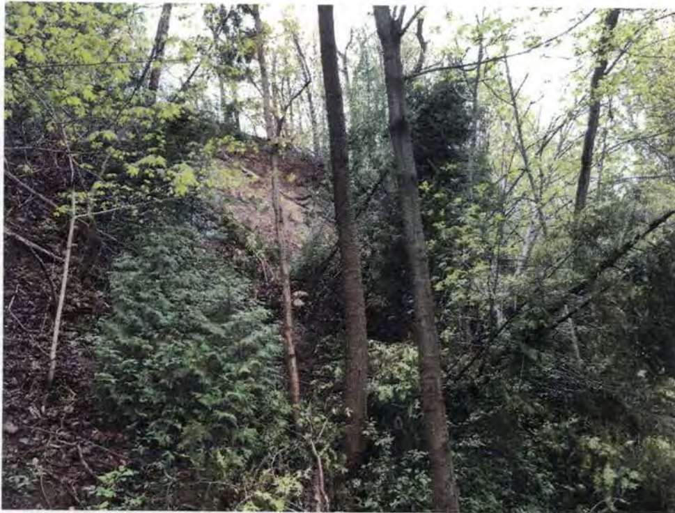
Sixteen Mile Creek Slope – Looking Northwest, slope overburden erosion, Cross Section B
