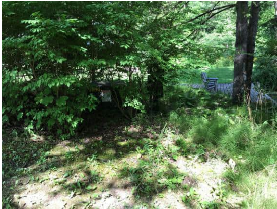
Picture 31: View of one (1) transformer located east adjacent to pond 2 (off-site) (July 20, 2020).
