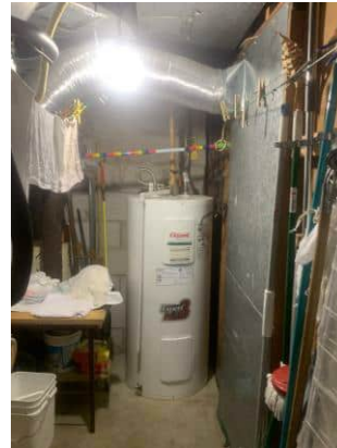
Picture 38: View of the propane powered furnace in the basement of 1350 Bronte residential dwelling (July 21, 2021).
