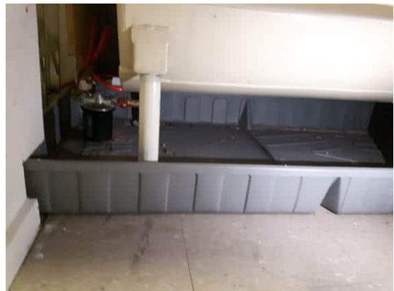
Picture 24: View of the AST at the basement of 1300 Bronte Road (July 31, 2020).
