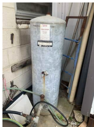
Picture 44: The pressurized water tank (used for irrigation of the garden) near the work shed at 1350 Bronte Road (July 21, 2021).
