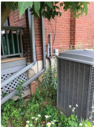
Picture 27: View of the vent pipes for the AST located at the basement of 1326 Bronte Road (July 20, 2020).
