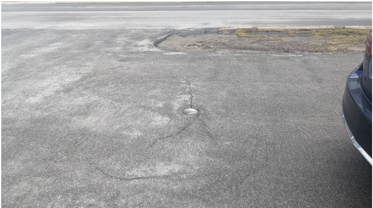
Photo of flush mount monitoring well located just south from the southeast corner of the Site building, facing southeast.
