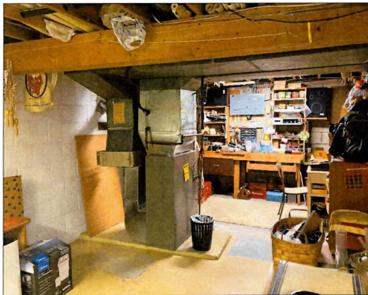
Photograph 10 – Current natural gas forced-air furnace on raised concrete pad in the basement.
