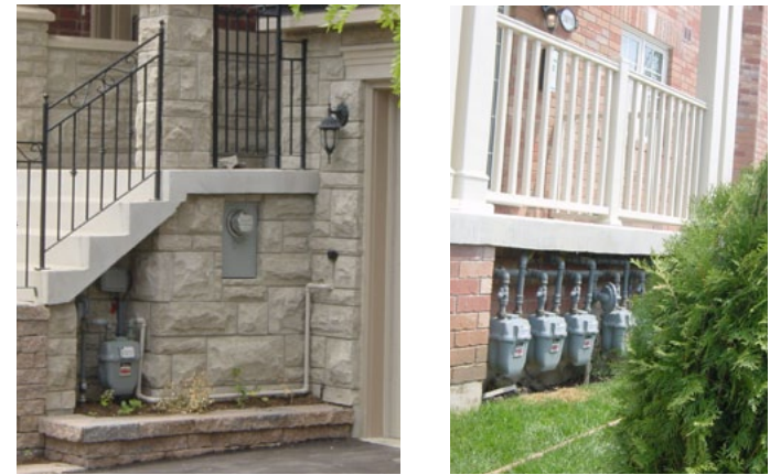
For townhouses and other higher density forms, utility meters should be architecturally integrated or screened
