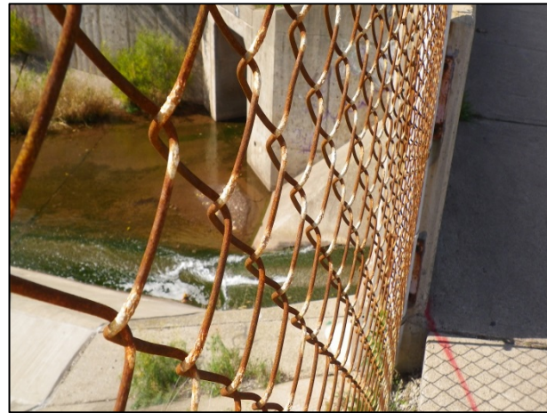
Morrison-Wedgewood Diversion Channel: Overlooking piped tributary that converges with main channel just west of Trafalgar Road (October 8, 2013).
