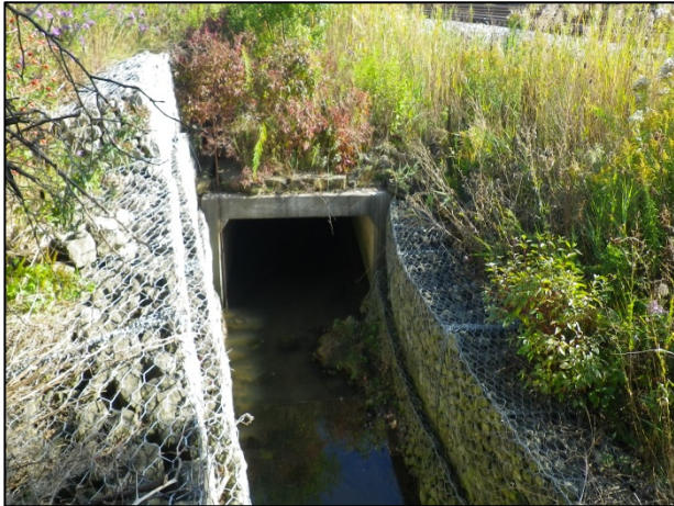
Tributary 1 of Lower Wedgewood Creek: Looking east (downstream), downstream of the convergence with tributary 2 (October 10, 2013).
