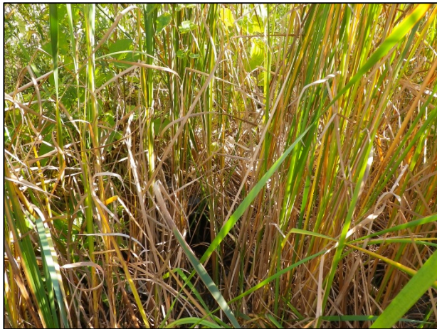
Ditch feature #1 of the QEW ditch system: Looking south (downstream) at the QEW crossing structure (October 8, 2013).
