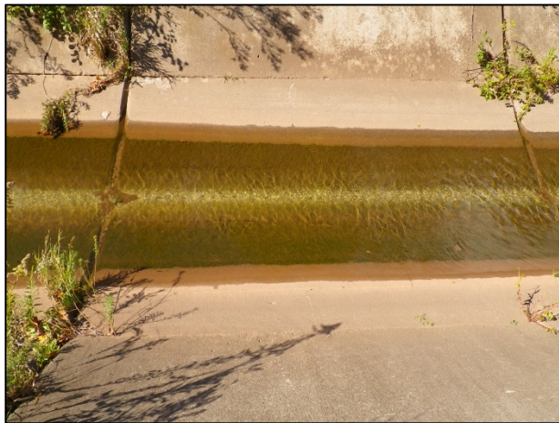
Morrison-Wedgewood Diversion Channel: Overlooking channel structure approximately 250 m east of Trafalgar Road (October 8, 2013).
